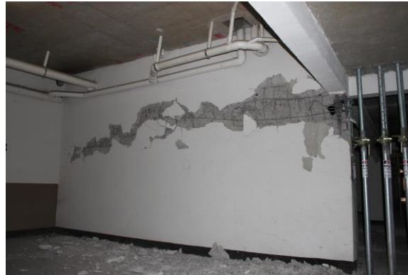
Fig. 1 – Sample image of reinforced concrete shear wall damage in the 2010 Chile earthquake [11-13]
